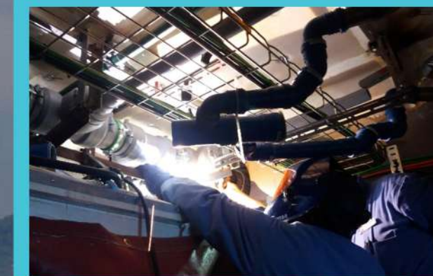
Replacement of the Coes Blue power grey water system to G.F piping in all the galley's drain
