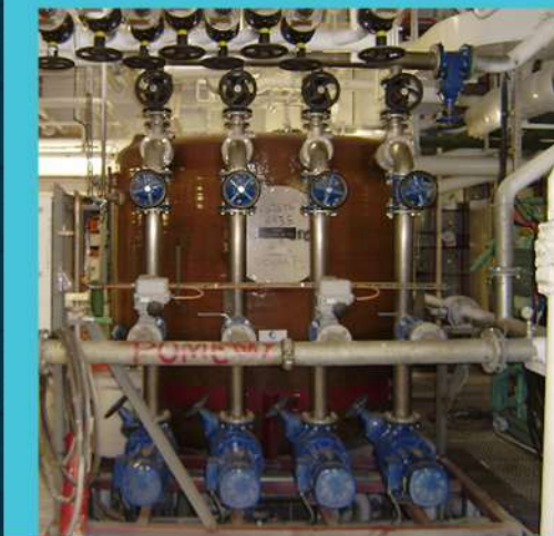
Replacement of the Evac vacuum toilet system to Jets vacuum toilet system
